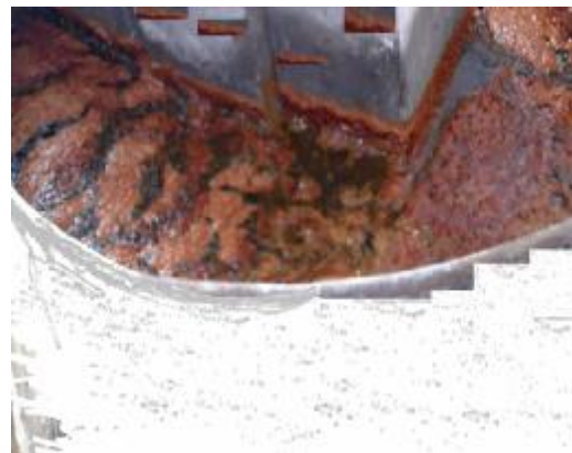
Figure 9. Photo for the beams during exposed to corrosion
