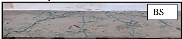
Figure 26. Crack Pattern for beam (BS) after 30 days of Corrosion Acceleration
