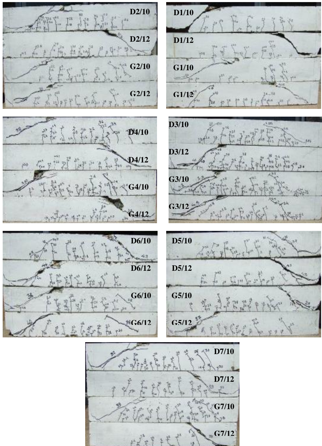
Figure 5. Cracking patterns at ultimate failure loads
