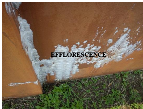
Fig. 1: Efflorescence on concrete wall.
