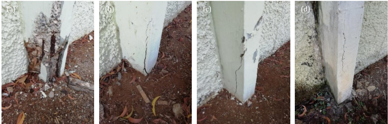
Fig. 2. Spallation of columns: a) C1; b) C2; c) C3; d) C4.
