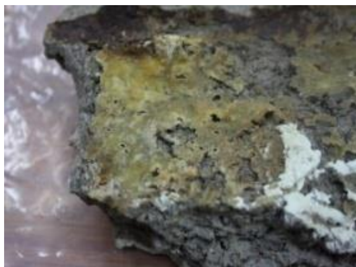
Fig. 8. Biogenic growth at the inner face of the column.
