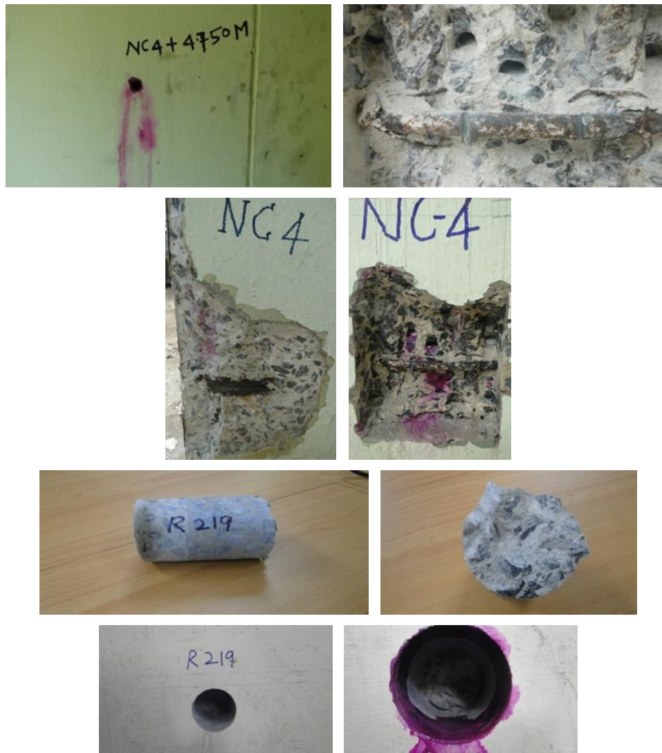
Fig. 7. Concrete carbonation tests on the fractured structural member, cored member and checking for the corrosion of rebar.
