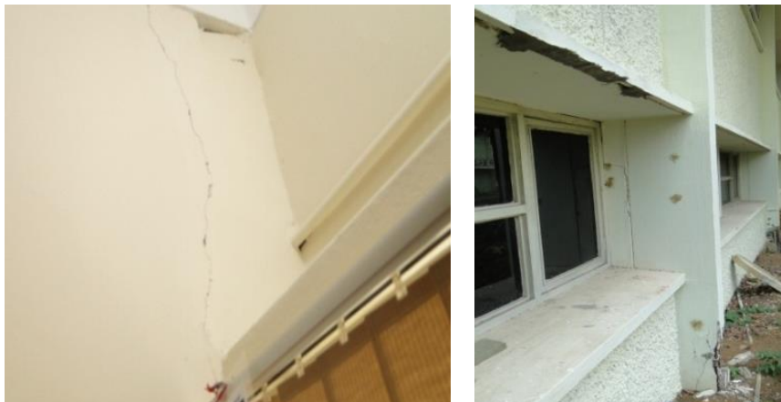
Fig. 3. Cracks in masonry and sunshades.
