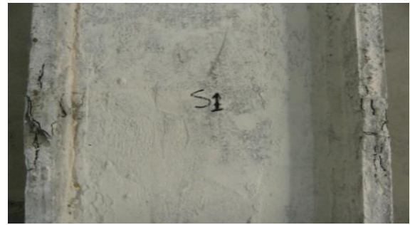
Crack pattern of S1
