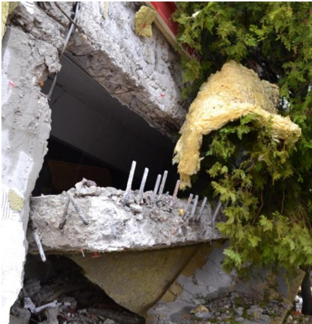
Fig. 1. Out-of-plane overturning and separation of an added reinforced concrete shear wall from the existing structure due to anchorage failure following the 2023 Kahramanmaraş earthquakes (Doğan and Karadağlı 2024).
