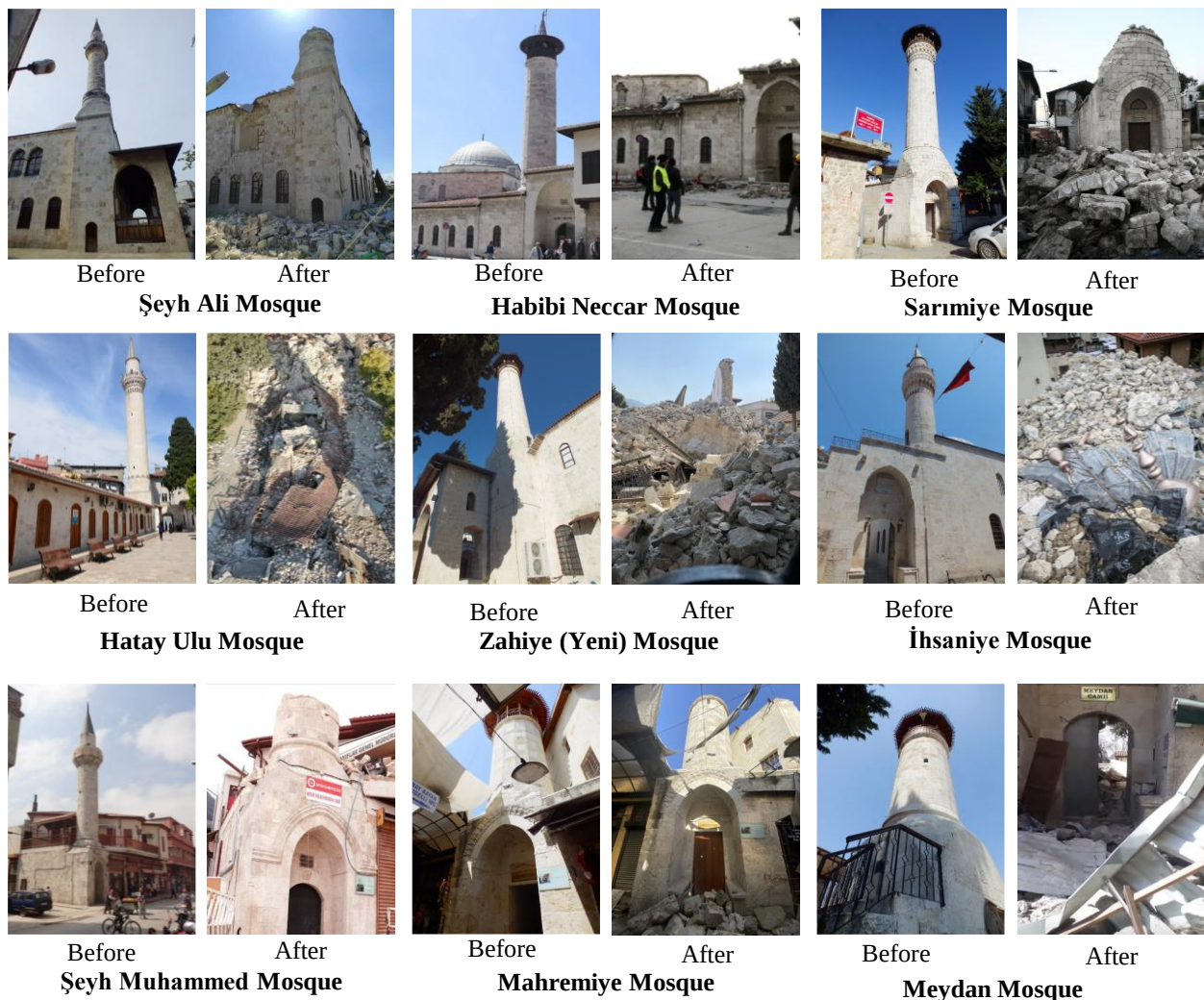
Fig. 1. Examples of historic masonry minarets damaged following earthquakes in Türkiye (Kocaman et al. 2025).
