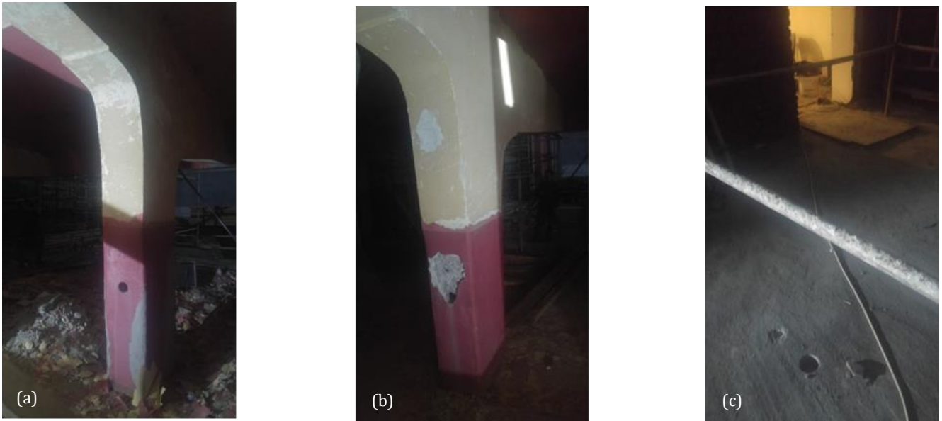
Fig. 4. Core samples taken from the structure: (a) Main column S41; (b) Main column S42; (c) Balcony flooring.
