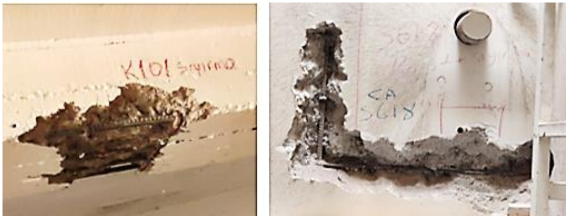
Fig. 2. Exposure of rebars.
