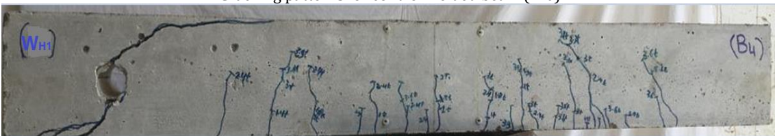
Cracking patterns for beam (WH1)
