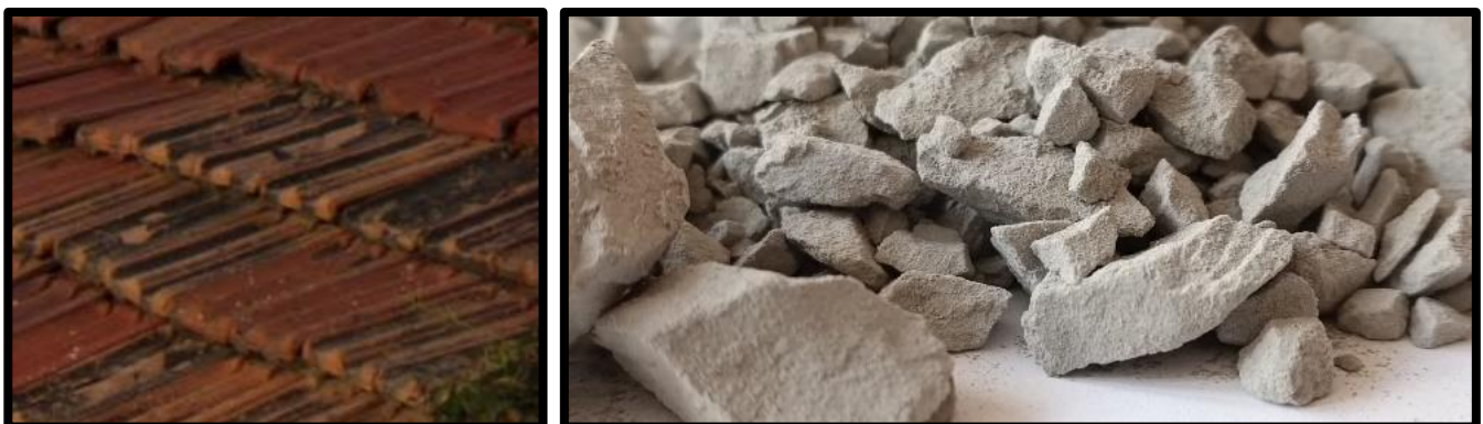
Fig. 1. Expired cement and aged roof tile.
