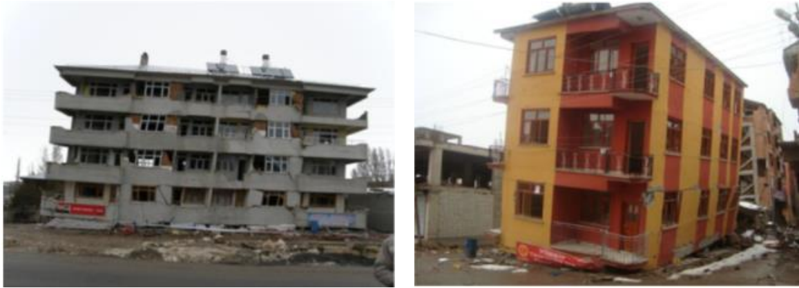
Fig. 1. Heavily damaged buildings whose ground storey columns collapsed due to the soft storey in the Van earthquake (Van Earthquake Report 2011b).
