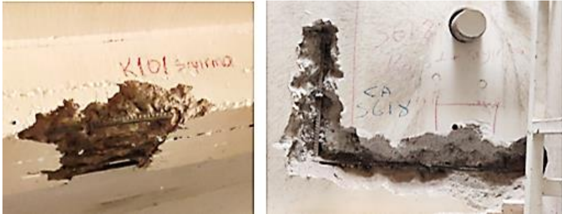
Fig. 2. Exposure of rebars.
