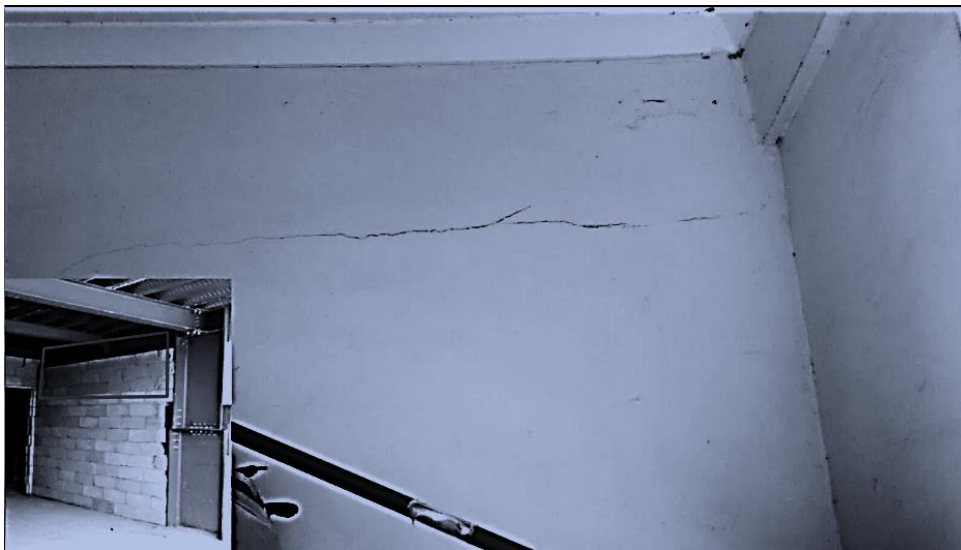
Fig. 4. Steel structure under construction and cracks between infill walls and steel frames.
